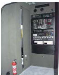
Rack & Door to Cab
