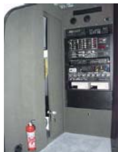
Rack & Door to Cab
